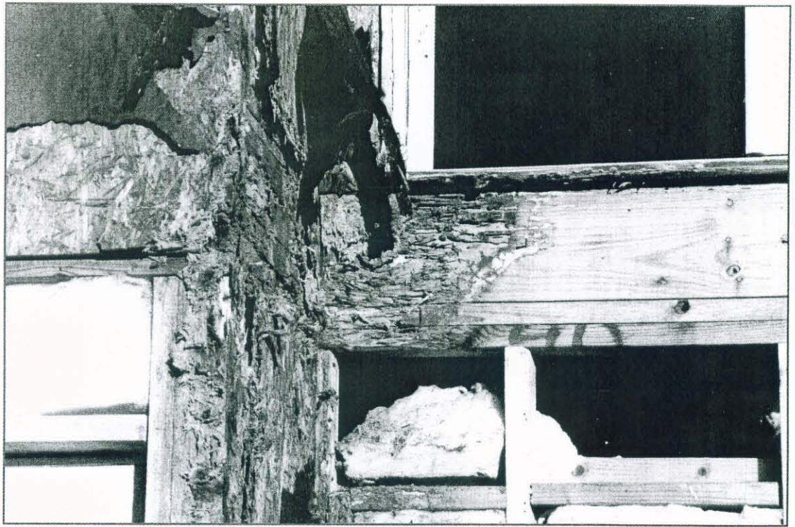
Photo 3: View of damages below a jamb/threshold intersection on a building clad with wood siding.
